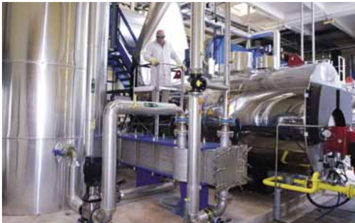
Energy eco-efficiency installation in the Vichy plant.
