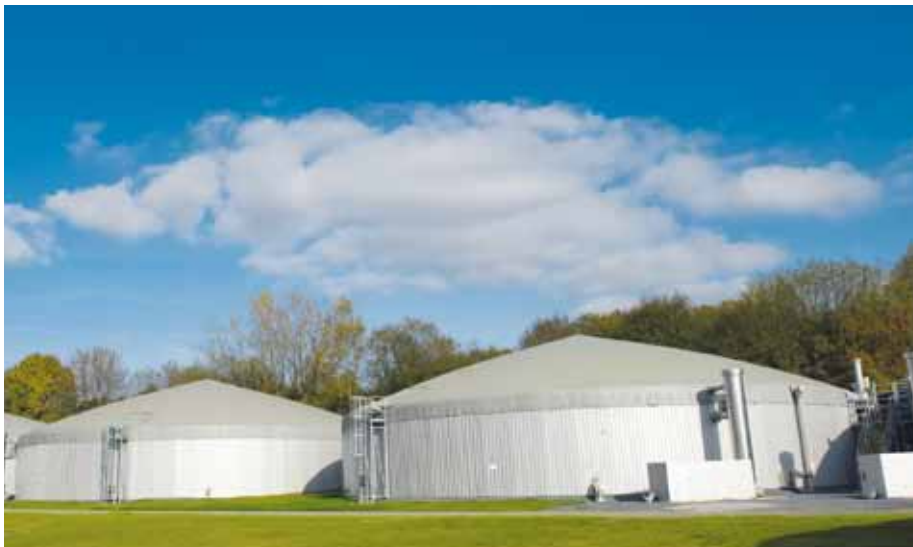
Bio-methanisation unit installed at the Libramont plant, the group's first plant to use 100% green energy.
